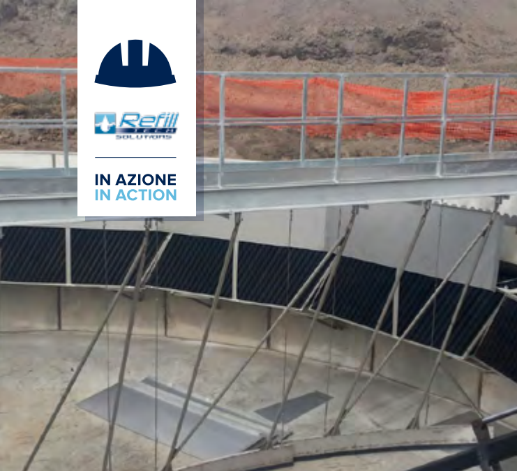
Sedimentatore circolare con LSM50 (PR) Circular clarifier tank with LSM50 (Parma - Italy)
